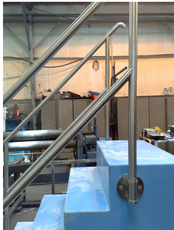
Double handrail on steps for Jordan Model
